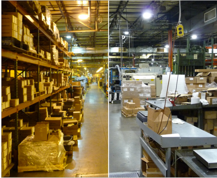
Figure 2: The Creed Monarch facility before (left) and after (right) installation of the Intelligent LED Lighting System from Digital Lumens.
